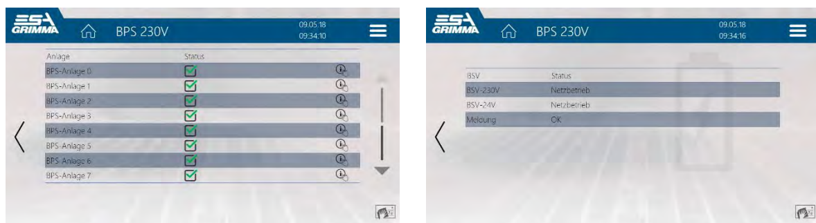
Fig. 10: left: trade overview “battery-supported power supply” right: trade view “battery-supported power supply”
